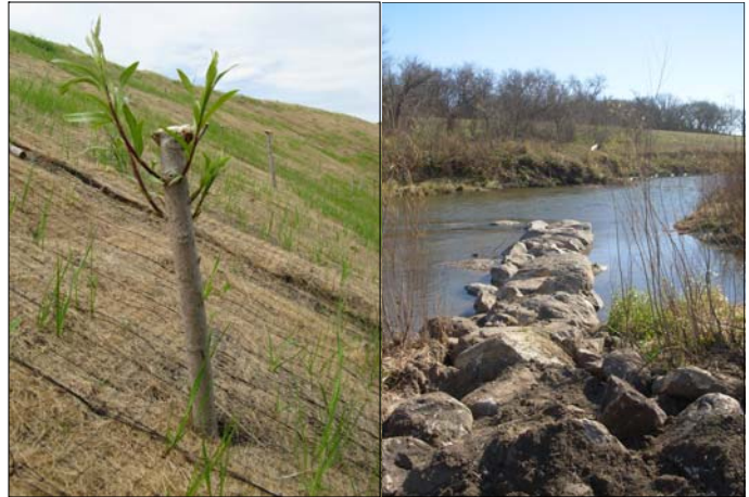
Willow stakes hold erosion control blanket in place & grow, too! Stream barbs help direct river current to middle of streambed & provide fish habitat.
